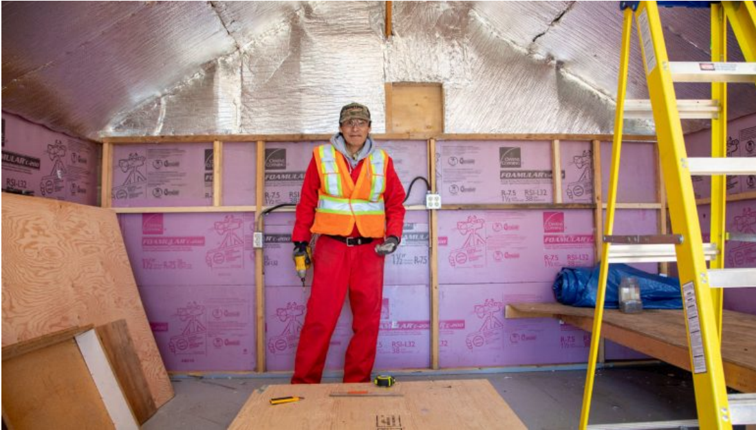
Archie Doctor, upgrading the accommodations at the Nechalacho camp. The structure will house additional employees planned to be hired when Cheetah's Rare Earth Demonstration Project starts production next year. (Photo courtesy of Bill Braden)
